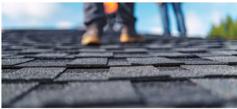
Your roof protects your home, your family, and your investment. Knowing when it's
