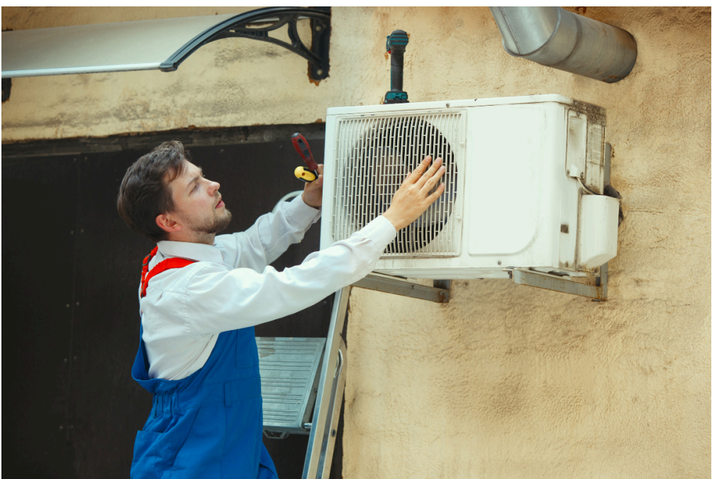
When a Tampa summer mid-day climbs up previous 95 and the moisture smothers everything it touches, a silent ac system sets off alarm system bells. If you live below enough time, you discover the indications before failing: a compressor that hesitates to start, provide vents that feel warm, a thermostat you keep pushing lower without alleviation. A/c is not a high-end in Hillsborough and
